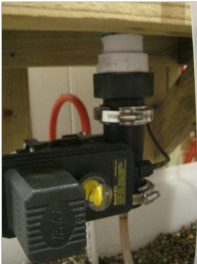
Figure A4. An image of an electronic dose valve placed directly under a dose tank.
