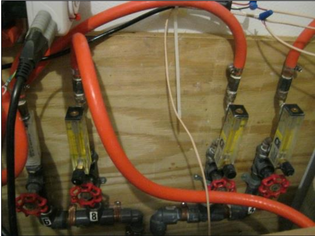
Figure A15. An image of the aeration distribution manifold.
